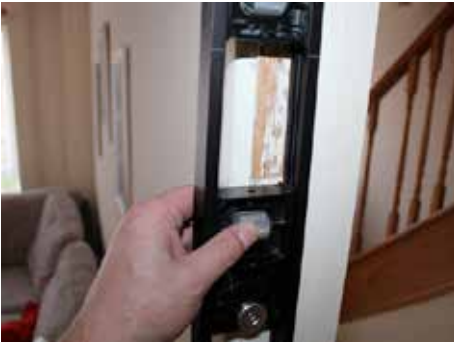
▲ The small lip on the right of the opening sits to the hinge recess
