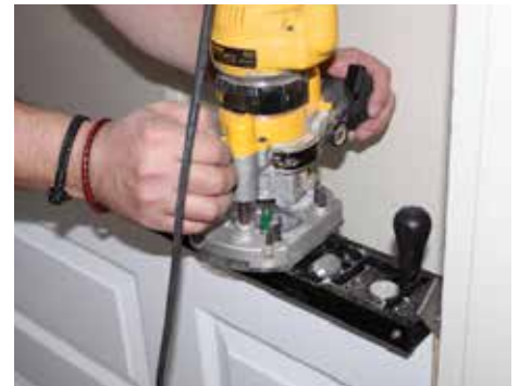
▲ The tab on the jig is hooked over the door to set the correct position before routing
